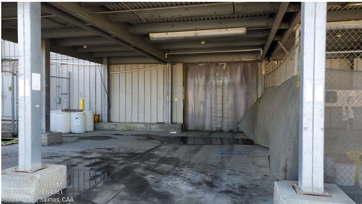
Photograph 2. View of the exterior hazardous materials storage area on the northern side of the 336 John Street building, with stained concrete and drums.
