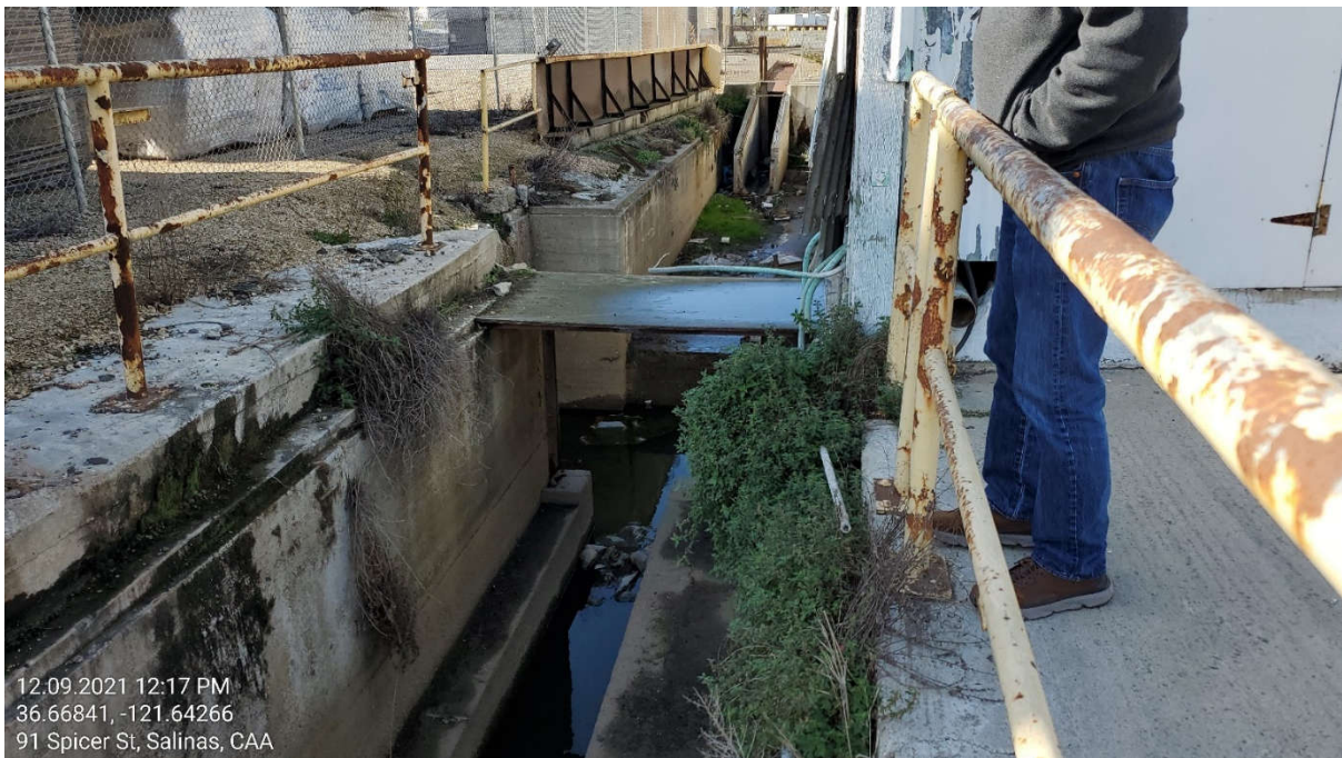
Photograph 6. View of an open portion of an industrial trench in the southeastern portion of the project site.
