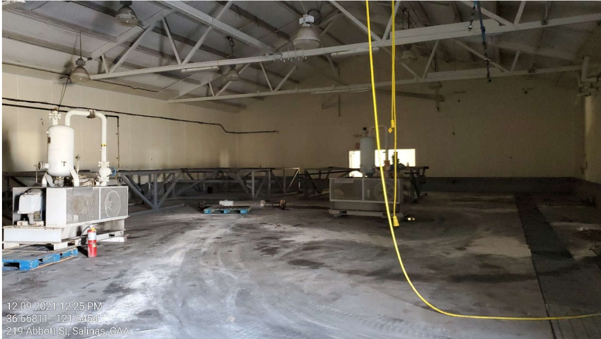
Photograph 1. View of the interior of the 239 Abbott Street building. Stained concrete and absorbent materials are visible.
