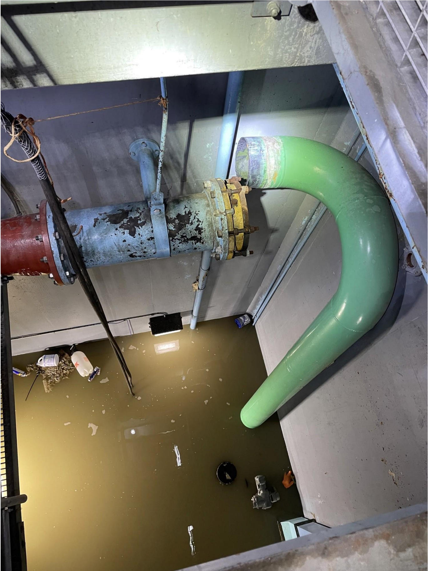
Image 3. Detached Pipe at Lift Station
