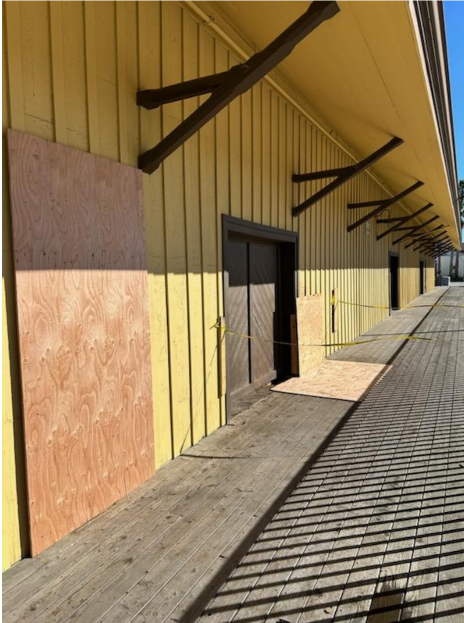
Fire damage at the California Welcome Center Building
