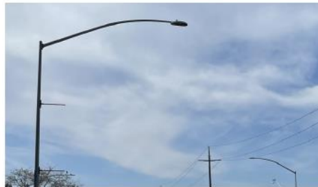
Caltrans standard cobra head for vehicular lighting. (Photo by: SWA)
