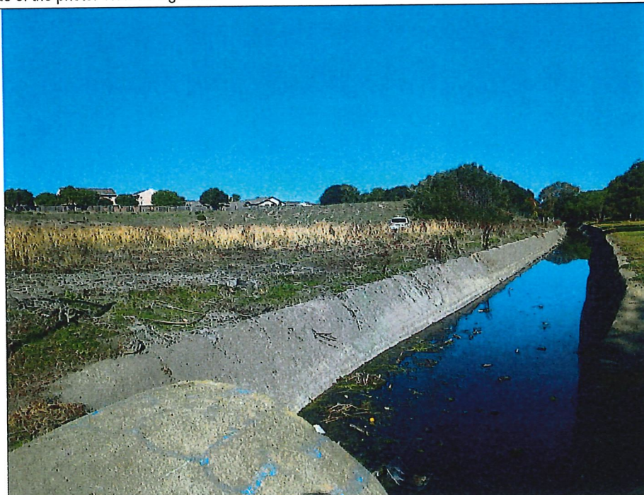
Photograph 2: (36.686279, -121.656684) View of the eastern portion of the project site with AR-01 in the foreground. View facing northwest.
